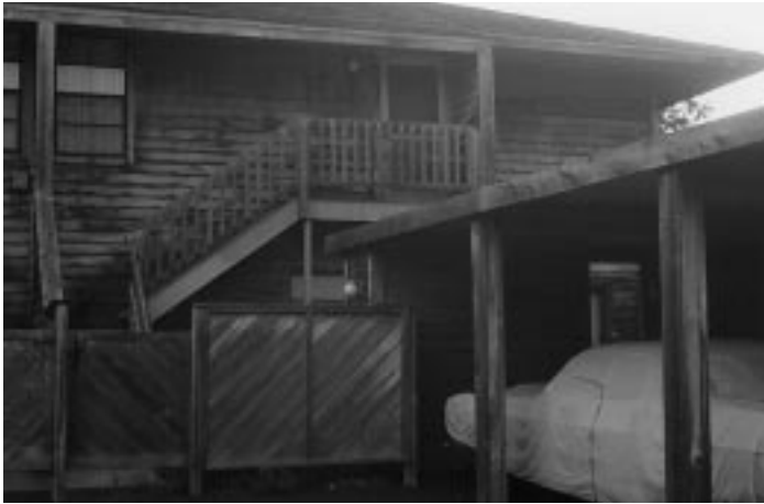
Before Cedar siding restoration
